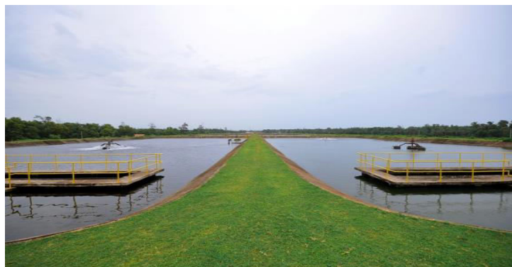
15 mld STP at Puri, Odisha
